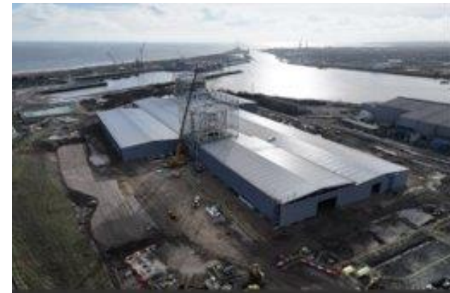
NEP1 – JDR Cables, Energy Central
